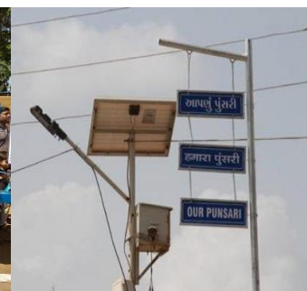
Figure 8 Punsari Solar Streetlight
